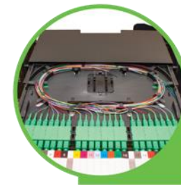
Large splicing area
